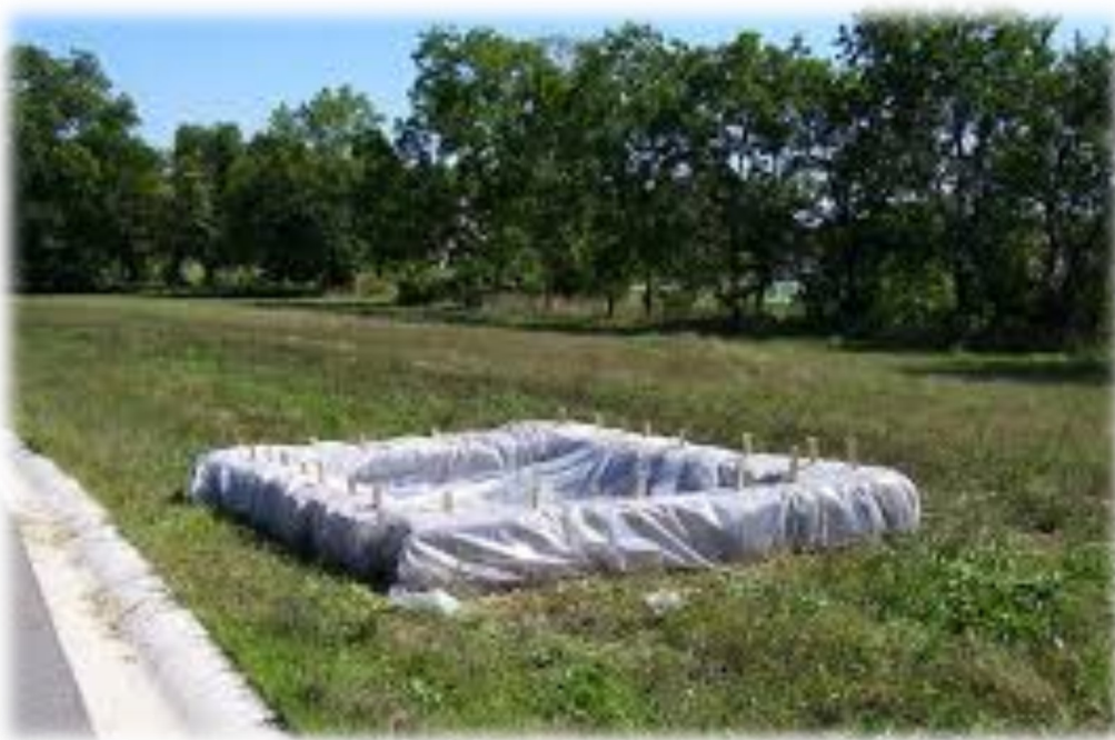
Temporary concrete wash out site preventing contaminants from entering the ground and the storm system.
